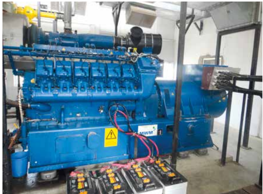
Picture 6: A view of installed power generation unit
