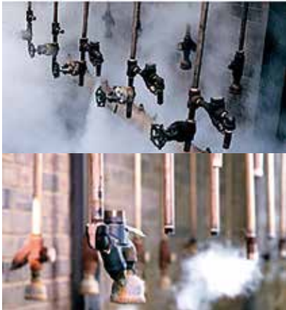
Picture 1: Reduction in loss from steam traps of high pressure system
