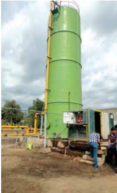
Picture 5: A visual of installed hydrogen sulphide biological scrubber
