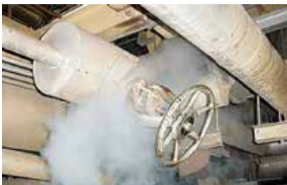
Picture 2: Steam leakage from valve
