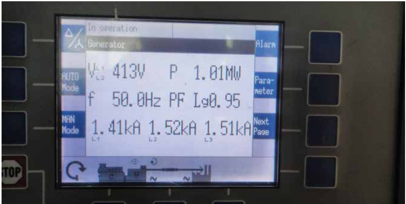
Picture 7: A view of control panel readings for power generation values
