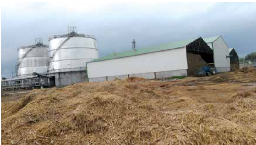
Picture 1: A view of paddy straw-based biogas plant installed at Fazilka, Punjab
